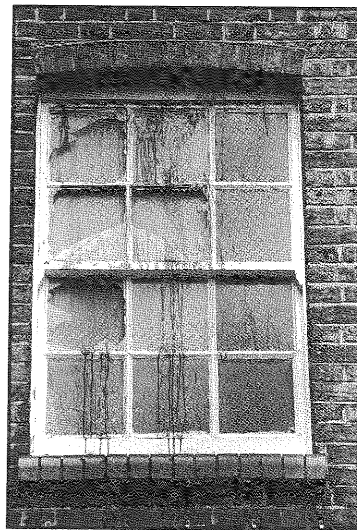
Blood-stained window. In an effort to escape a racist arson attack, one of the occupants smashed windows with his bare hands
